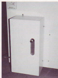
W: Automatic water supply
